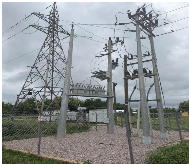
Installed Capacitor Banks at Bimbilla
