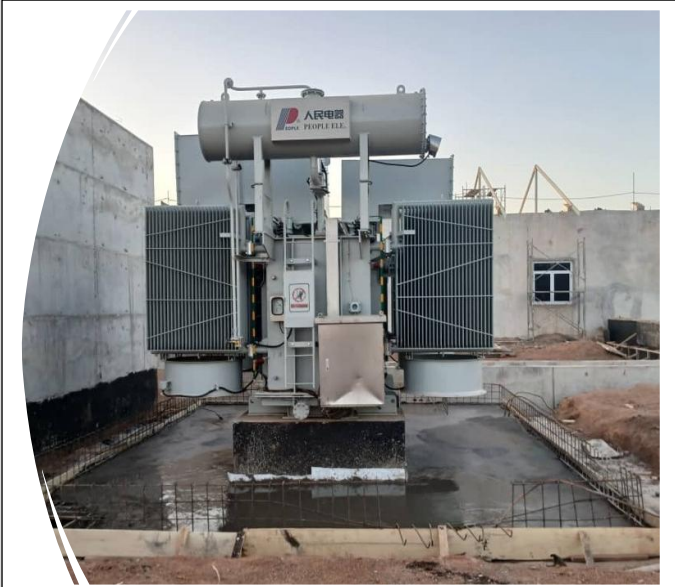
Sample of installed 20/26MVA Power Transformer at Lamashegu
