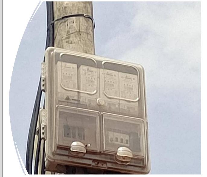
Samples of installed smart split prepaid meters
